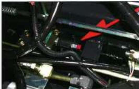
• Electromagnet check valve (plot plan drawing C) (For prevention from drop of the mower #1, #2, #3, #4, #5)
